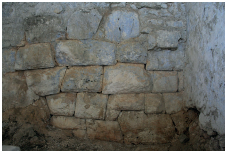
Fig. 5. The Hellenistic wall within the St Mary of Cassiopitra church (photo K. Çipa)
